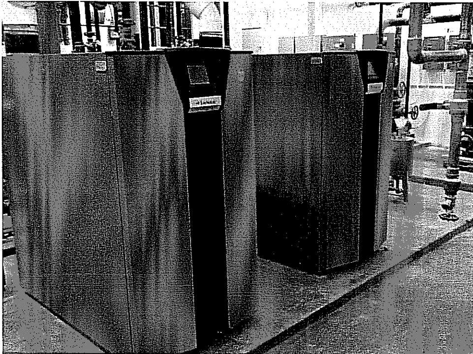
ABOVE: Middle School Boilers AFTER
