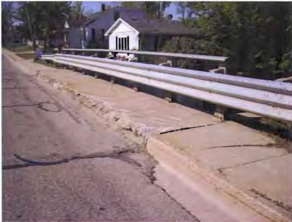
Deterioration of Curb/Sidewalk
