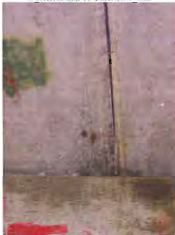
Cracking of Beam underside and Rust Stains
