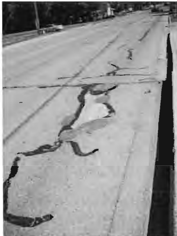
View of typical cracking and patch on Bridge Surface
