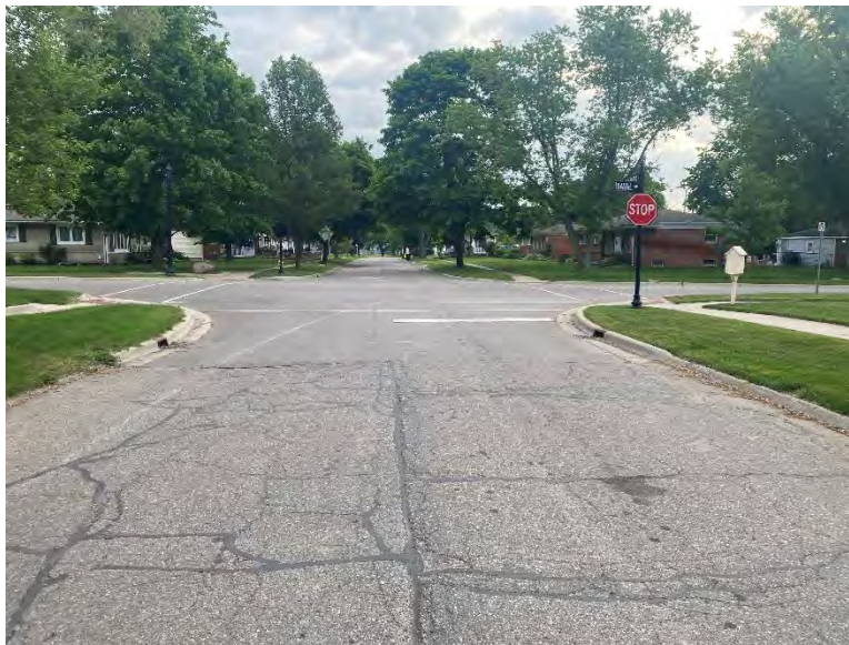
Don Shenk Drive @ Duval Drive looking Northeast.
