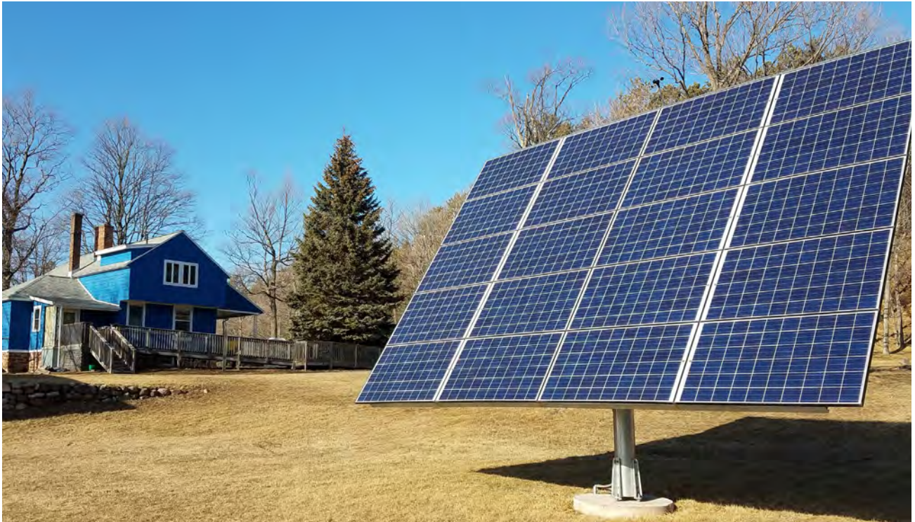
Ground-mounted monopole SES. Photo by Bradley Neumann.
