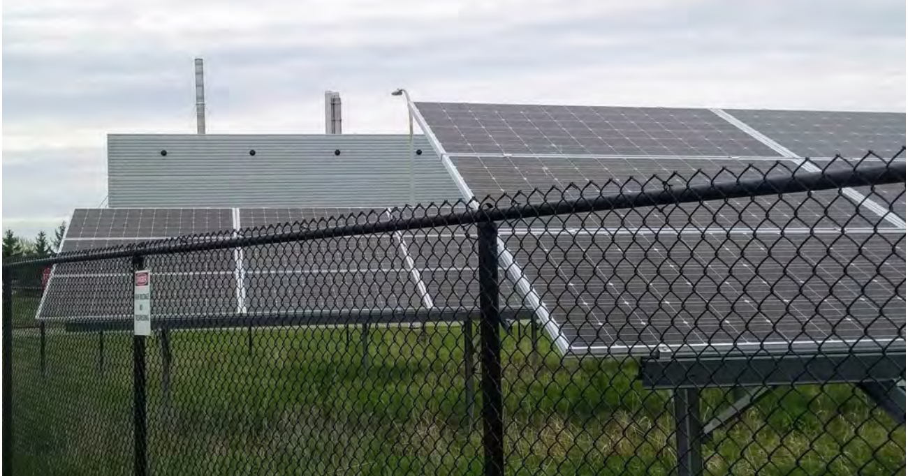
Consumers Energy - Western Michigan University, Business Technology and Research Park solar garden. Photo by Mary Reilly.
