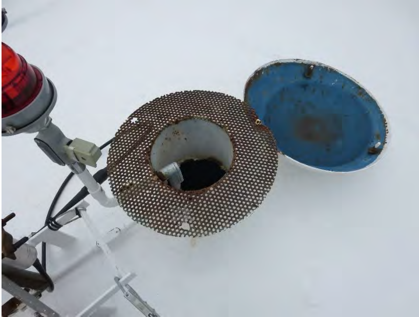
PHOTO #1: As found on inspection
